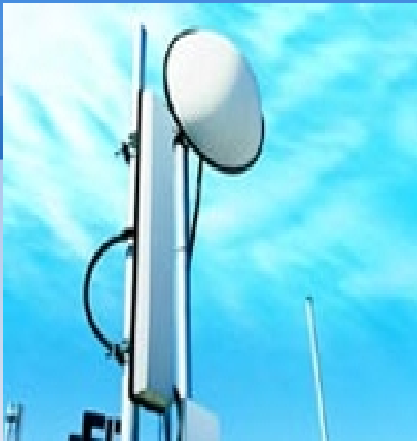
A WIMAX tower
